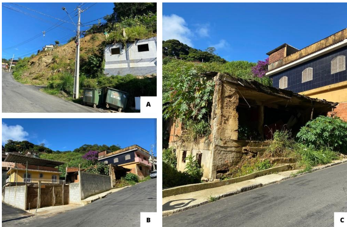
Figure 6 – Chácara Flora, 01 year after the disaster of 15 February, 2022 (18/02/2023). A) Destroyed houses hanging on the slope; B) Destroyed houses near Centro de Educação Infantil Deise Elói Gomes; C) House affected at the base of the slope
