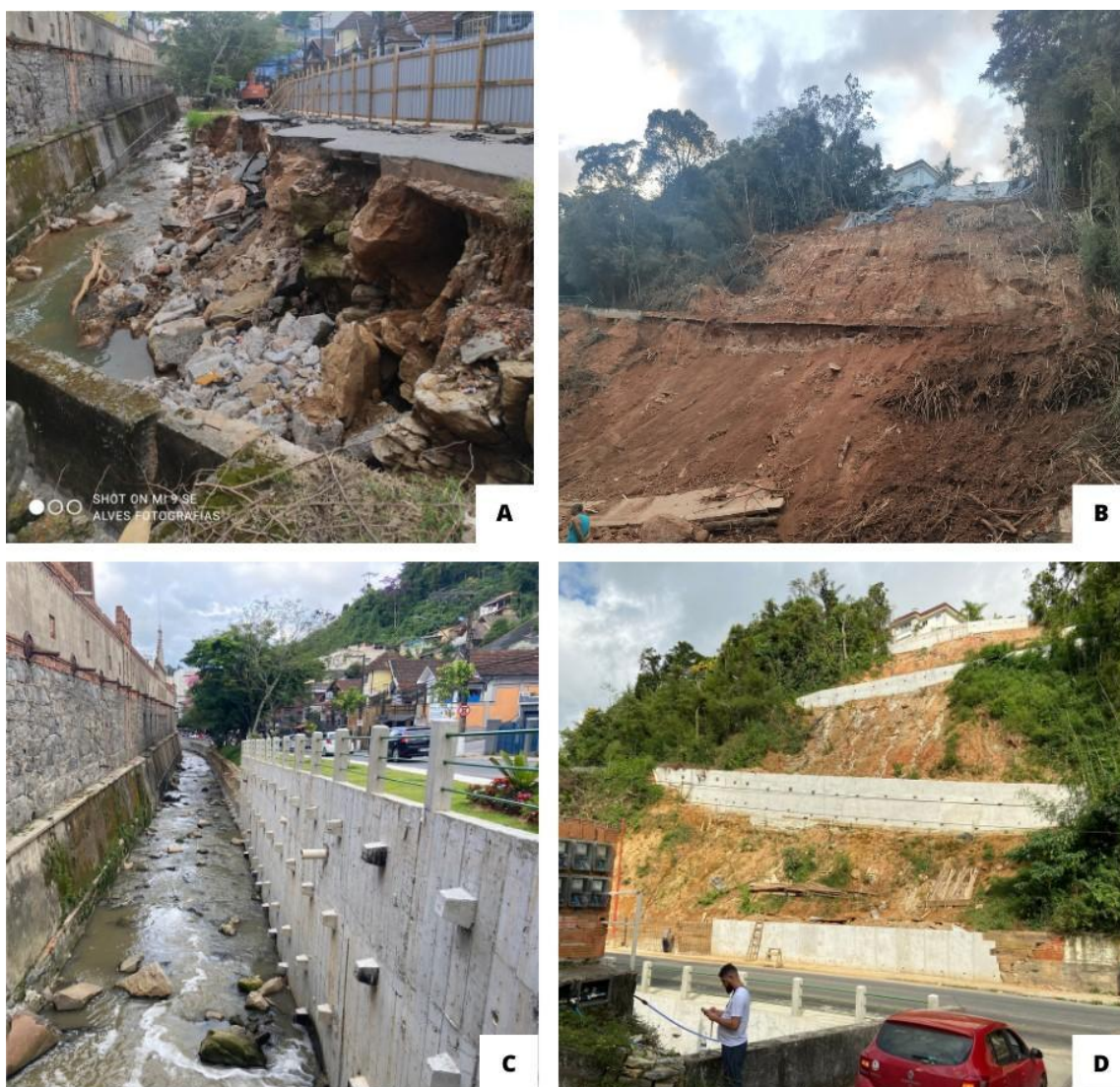
Figure 9 – R. Washington Luiz: A and B) 39 days after the disaster on 15 February, 2022 (26/03/2022); C and D) one year after the disaster (18/03/2023).
